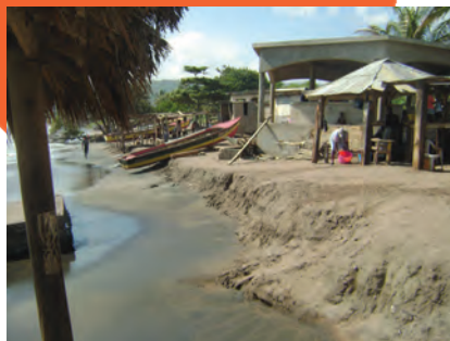
More intense hurricanes and rising sea levels will contribute to coastal erosion in many Caribbean countries. Photo: Stephen Smalling
