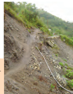
Landslide in Cascade Jamaica. Photo: Jamaica Conservation and Development Trust.
