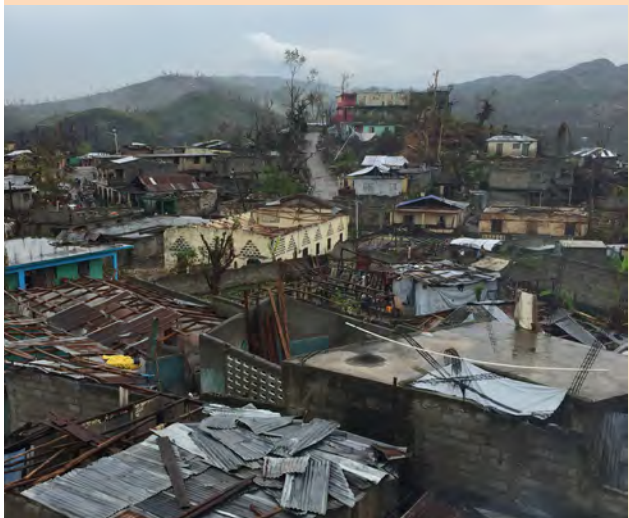
Figure 10: Damage in the city of Moron, Haiti, following Hurricane Matthew. Photo: Avi Hakim, CDC (Flickr) [CC BY 2.0 ( http://creativecommons.org/licenses/by/2.0 )], via Wikimedia Commons
